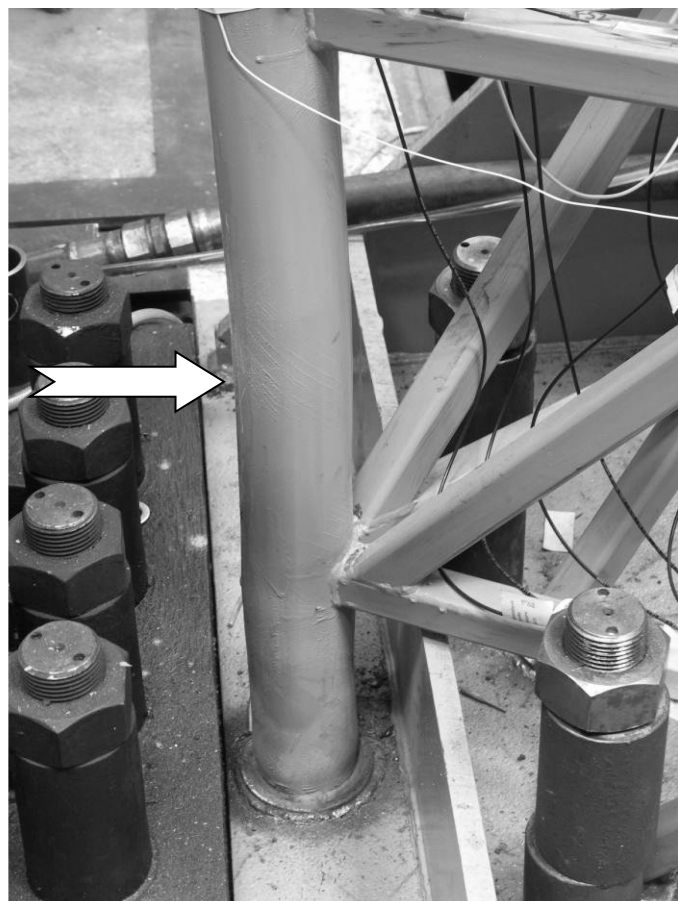
Figure 6. Bottom part of chord A after yielding.
