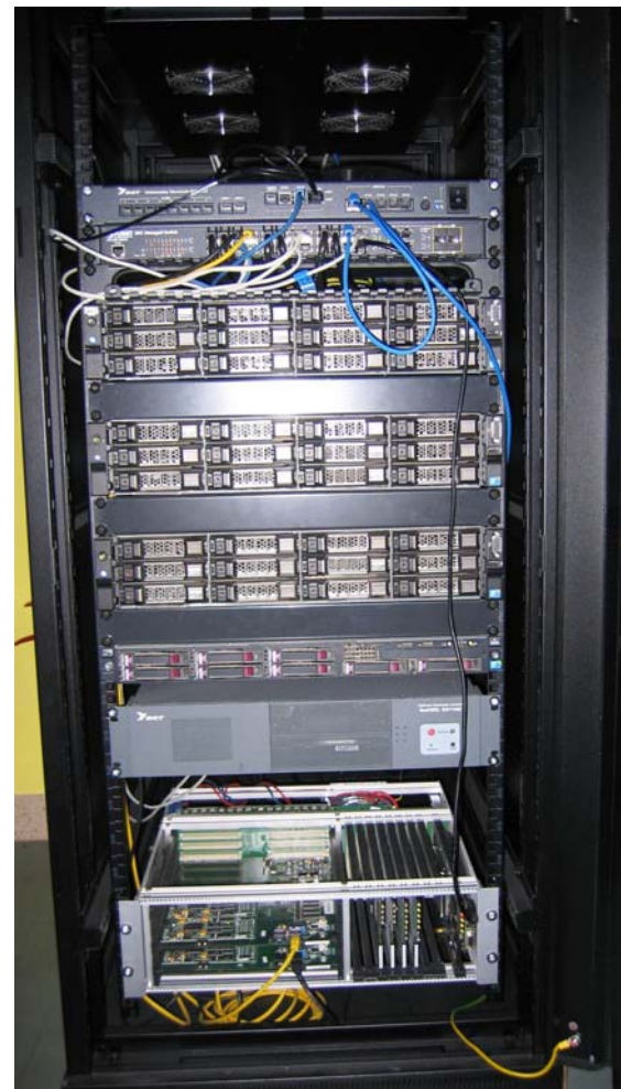
Figure 2. From the top: URC for OP, switch, Archive Servers (AS), voice recorder, telephone server.
