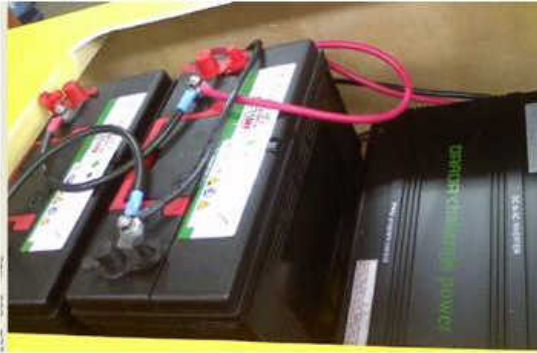
Figure 1. Battery and converter
