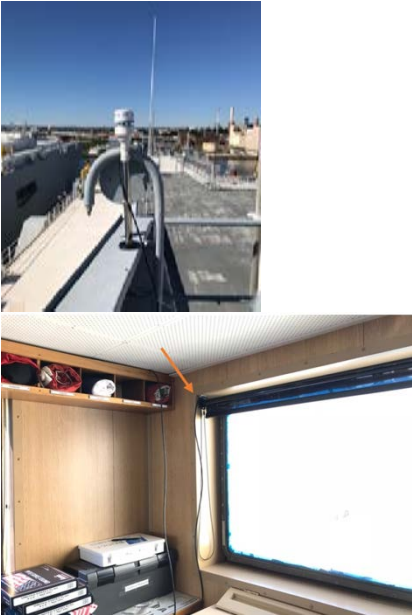
Figure 5. Airmar weather station mounted to rail (left) and cable coming through stuffing tube to bridge (right).
