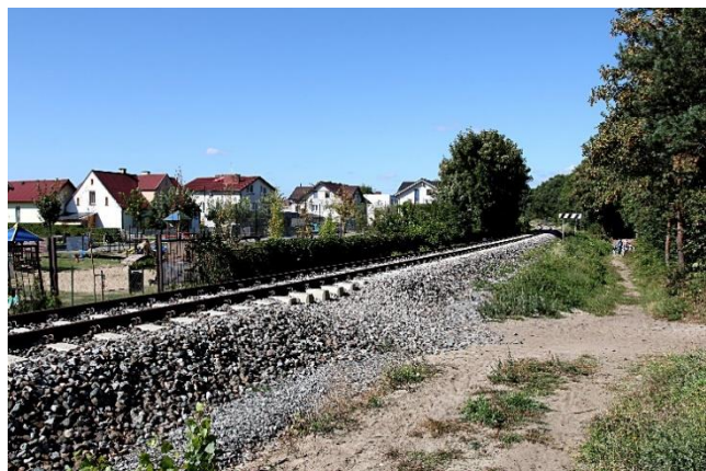
Figure 6. Defects in the ballast at an illegal track crossing
