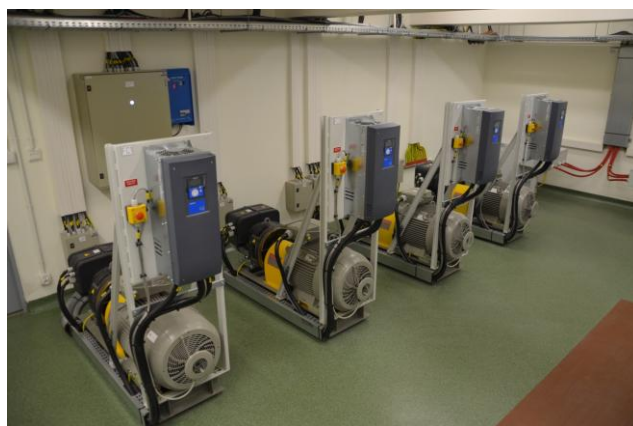
Figure 4. Generator sets: G1, G2, G3/M and SG placed in GSR C010
