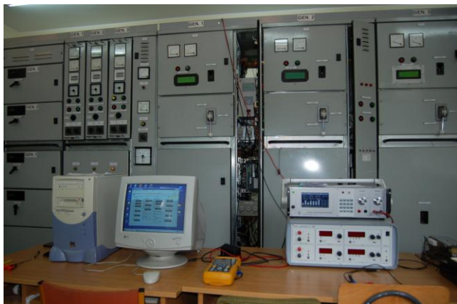
Figure 2. Historical didactic room with the main switchboard
