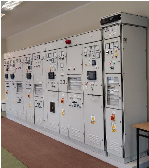
Figure 5. Main switchboard 3x400 VAC and 3x230 VAC, 50Hz
