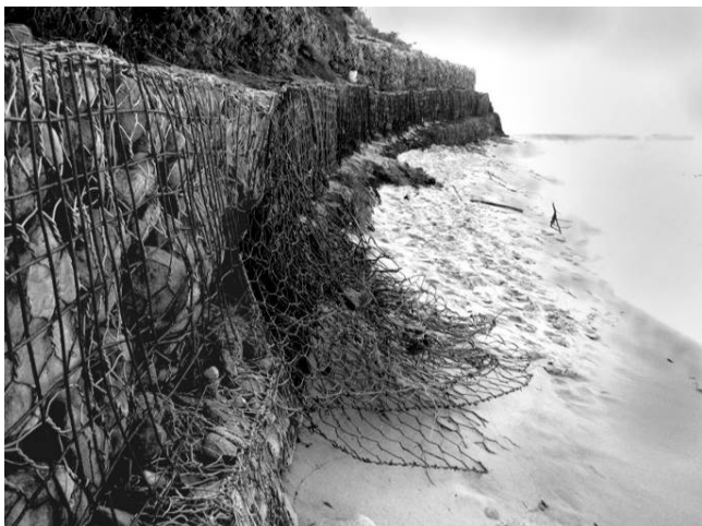
Figure 8. Example of poorly effective coastal protection: partly destroyed gabions at Jastrzebia Góra (photo by the author).
