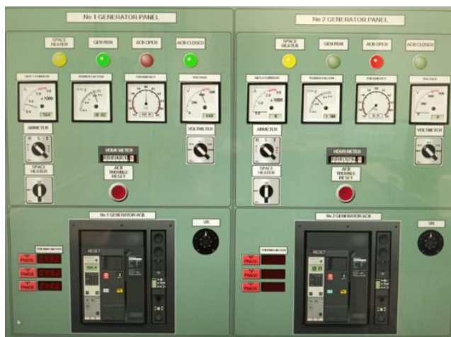
Figure 3. Generator Panels of a Dual-Fuel Tanker Ship on Wärtsilä Engine Room Simulator at UNIGE
