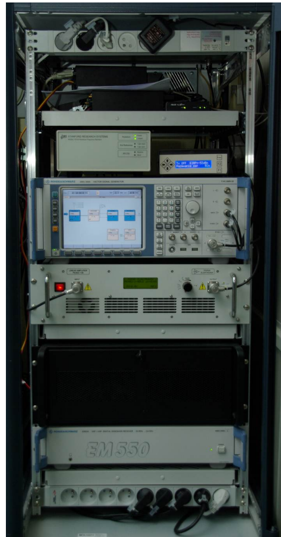
Figure 9. Hardware implementation of a Master station
