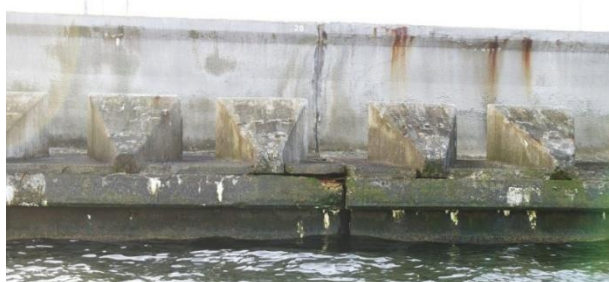
Figure 5. Case study 2, View of the expansion chamber from the bay side: visible damage to the superstructure (exposed reinforcement) and wave deflectors, as well as rust stains caused by reinforcement corrosion and concrete loss in the area of the structural expansion joints, source: own
