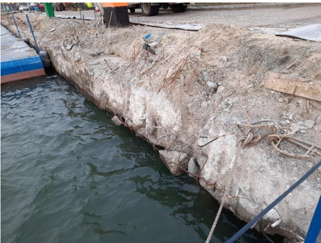
Figure 15. Case study 5, Quay condition before renovation, showing significant concrete losses and exposed, corroded reinforcement wall, source: own
