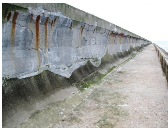
Figure 6. Case study 2, View from the expansion chamber; visible surface damage to the breakwater parapet following previously conducted repairs, source: own
