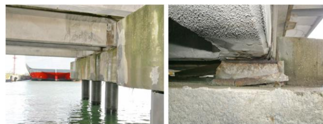
Figure 12. Case study 4, Condition of the platform before renovation. Visible severe damage to both fixed and unidirectional sliding bearings. Extensive corrosion is observed on both steel and elastomeric components. Bearing pedestals are heavily degraded, with numerous cracks, material losses, and spalling, source: own
