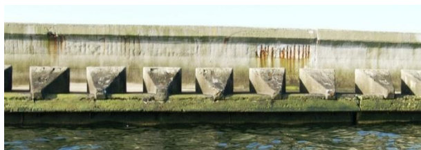
Figure 4. Case study 2, View of the expansion chamber from the bay side: visible surface damage to the wave deflectors and exposed reinforcement of the breakwater parapet, source: own
