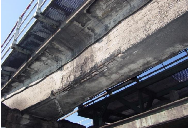
Figure 18. Case study 6, Bottom layer of the beam - visible delamination of the reinforcement cover, exposed reinforcing bars, source: own
