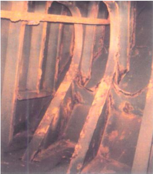
Figure 3. Coating in FAIR condition [20]
