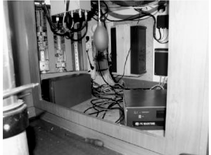
Fig. 5. Boxes and wiring
